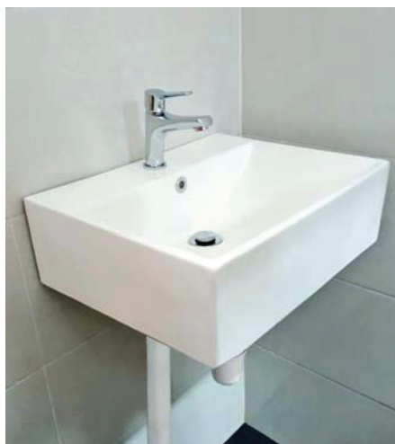
Wash basin with tap mixer
