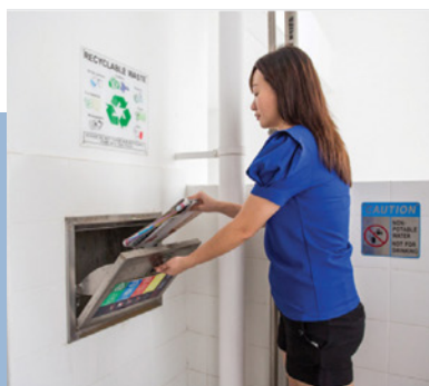
SEPARATE CHUTES FOR RECYCLABLE WASTE
