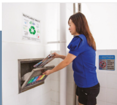
SEPARATE CHUTES FOR RECYCLABLE WASTE
