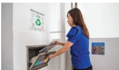
Separate chutes for recyclable waste
