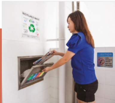
SEPARATE CHUTES FOR RECYCLABLE WASTE
