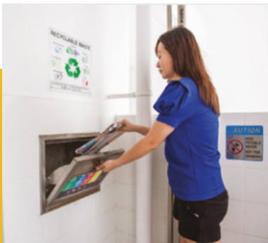
SEPARATE CHUTES FOR RECYCLABLE WASTE
