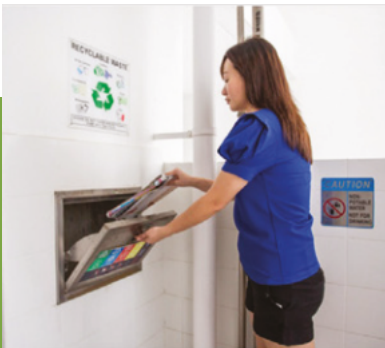
SEPARATE CHUTES FOR RECYCLABLE WASTE
